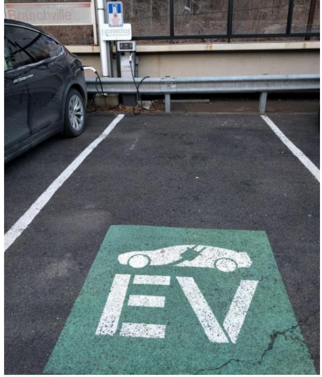
Branchville EV charging station
