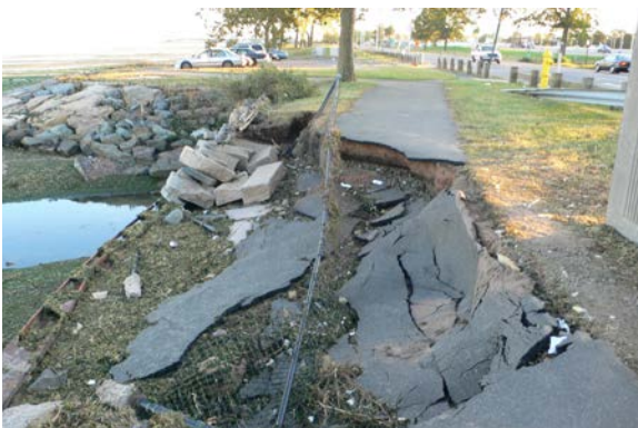
Shoreline Erosion at Long Wharf Park due to Hurricane Irene.
